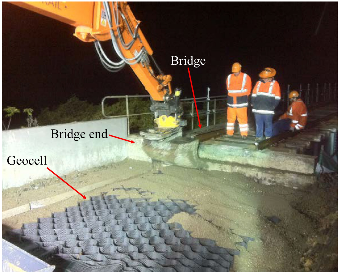
Figure 6.4 Installation of geocells at the railway bridge ends on the south coastline of New South Wales, Australia
