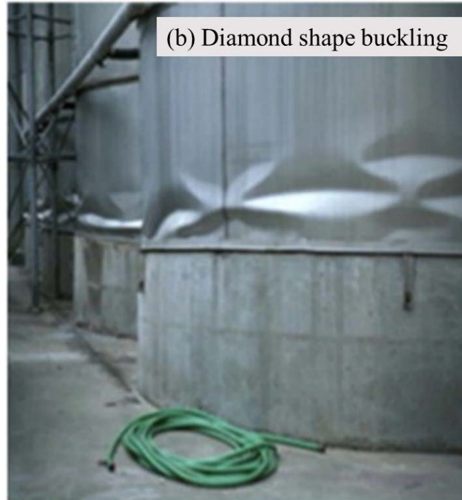
Figure 2.12 Observed damage for steel tanks under seismic load (a) elephant foot buckling example, and (b) diamond shape buckling (Malhotra et al. 2000)
