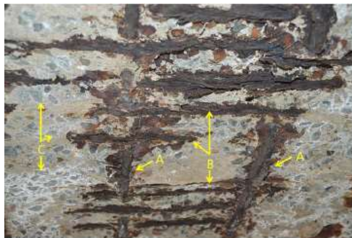
Figure 1-2. ASR and chloride-induced corrosion combined effects. (A) corrosion of prestressing strands, (B) corrosion of stirrups and (C) white ASR gel deposits (Berndt, 2019)
