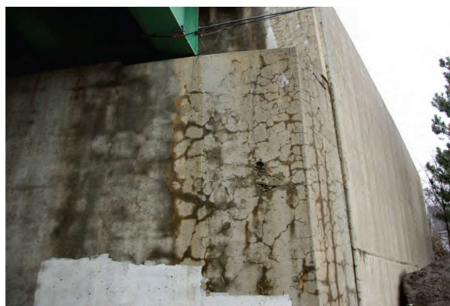
Figure 2-6 ASR is much more severe on the right side of the bridge abutment where it is exposed to environmental conditions, the left part covered by the bridge deck has minor ASR cracking when compared to the right side (Thomas et al., 2011)
