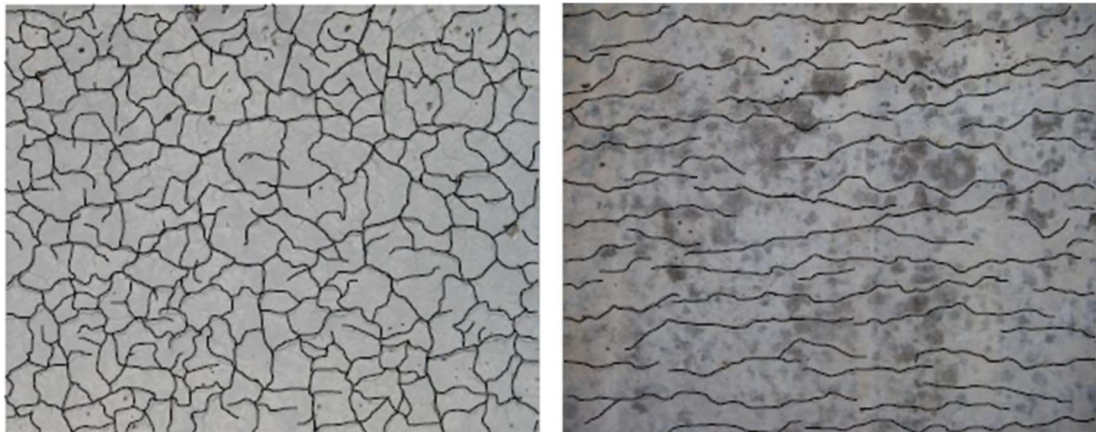
Figure 2-8 Orientation of cracks in reinforced and plain concrete: Map cracking on the left picture and cracking in the direction parallel to the rebar in the reinforced concrete on the right (Kreitman, 2011)
