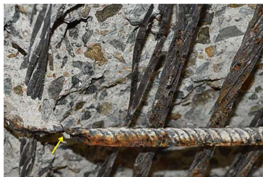
Figure 2-17 Corrosion of stirrups and prestress strands with heavy stirrup corrosion at the bending location (Berndt, 2019)
