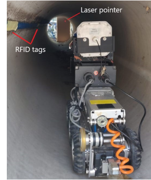
Fig. 2: Robot inside a pipe.
