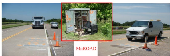
Figure 88: Installation of CNT/cement sensor in roads for testing monitoring capability (Rana et al. 2016)
