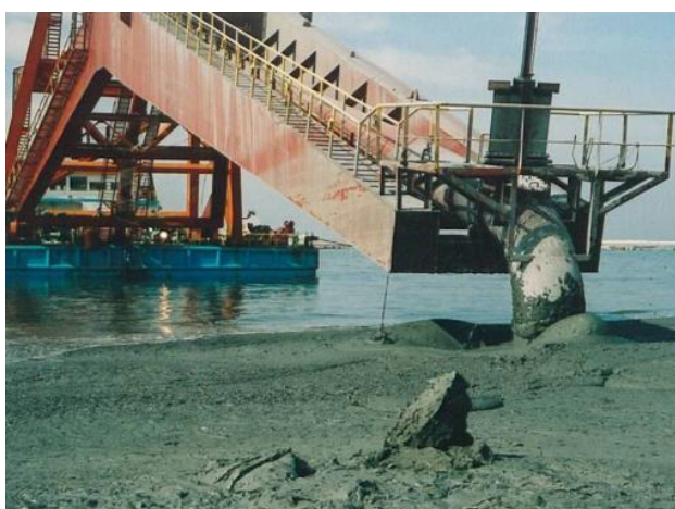
Figure 10 Cement treated dredged clay method was used for the reclamation of the site (Courtesy Prof Yoichi Watabe).
