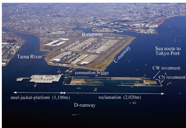
Figure 11: Aerial view of construction site and existing airfield on March 15th, 2009 (Courtesy Prof Kitazume).
