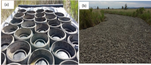
Figure 86: A view of the reinforced access track at Ballina site: (a-b) before and after infilled with crushed rock (unpublished part of a current program at the University of Technology Sydney through funding from the Australian Research Council, courtesy Ms. F. Mehmood, PhD student)
