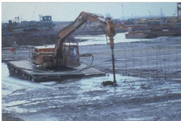
Figure 6 To enable trafficability, a shallow solidification method was conducted with heavy machine on a barge (courtesy of Kanto Regional Development Bureau, MLIT, Japan).
