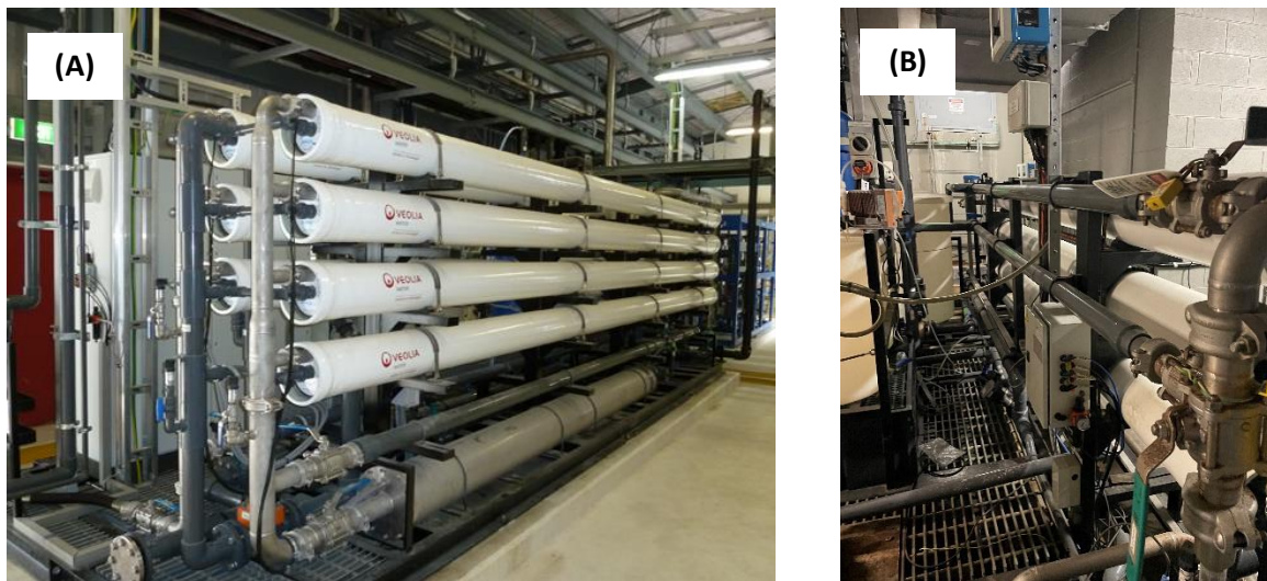
123 Figure 1: (A) A typical off the shelf packaged RO system for industrial application, and (B) 124 The packaged RO system for sewer mining at Darling Quarter (Sydney, Australia).
