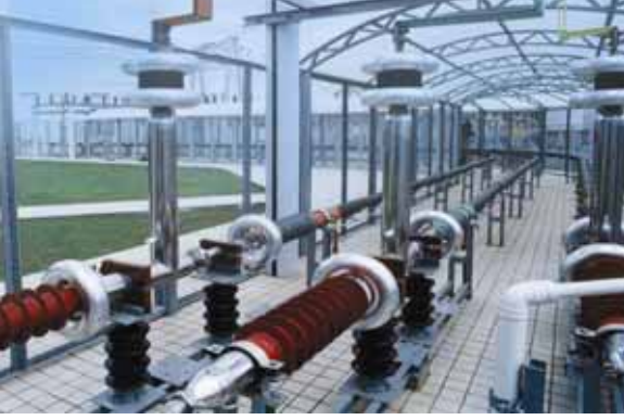
Fig. 1. HTS cable site at Puji substation in China.
