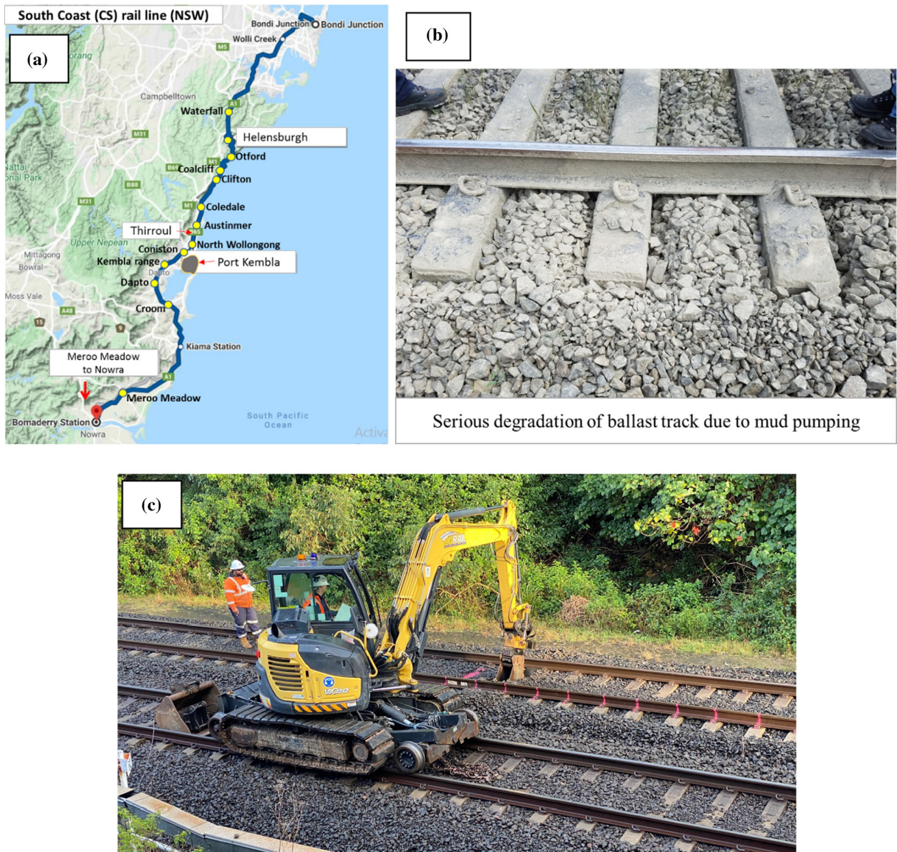
Fig. 2 Site investigation on mud pumping rail tracks: a map of the South Coast Illawarra (SC) rail line with bog hole locations, b severe fouling of rail track due to mud pumping, and c excavation and sampling
