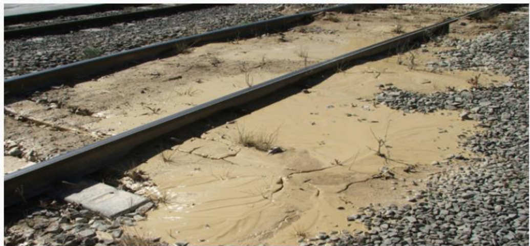
Fig. 1. 3 Mud pumping of saturated subgrade soil (Picture Courtesy: Professor Buddhima Indraratna)
