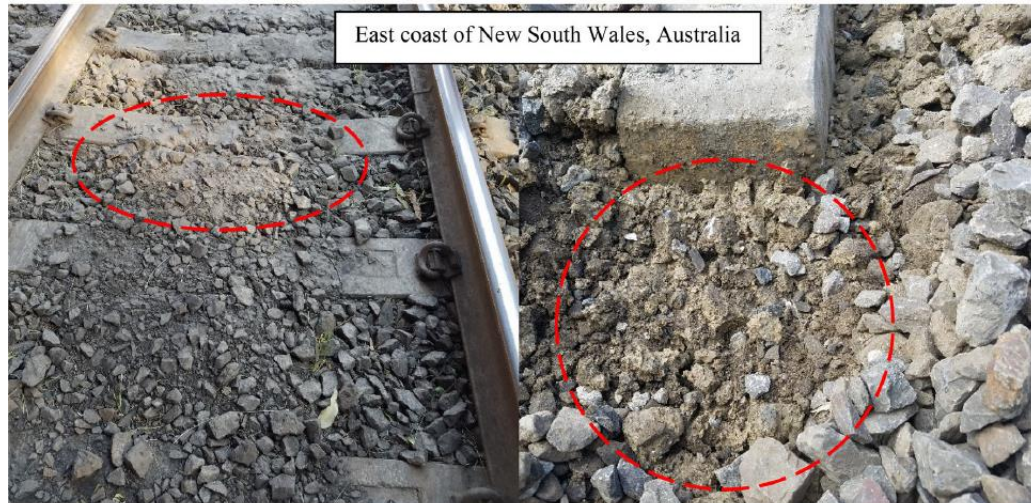
Fig. 2. 2 Mud pumping occurred along the east coast in NSW, Australia (Picture Courtesy: Prof. Buddhima Indraratna)
