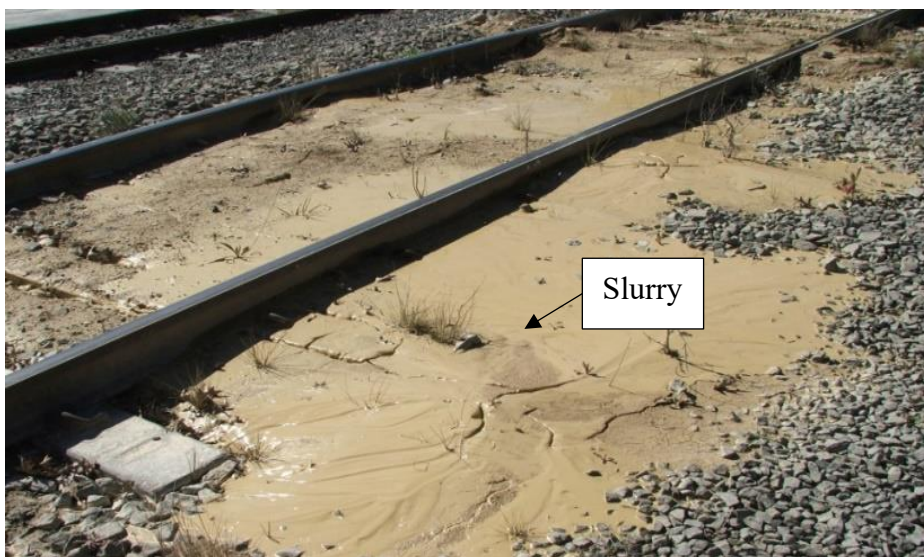
Figure 1. 1: Subgrade mud pumping (Courtesy: Prof. Indraratna)
