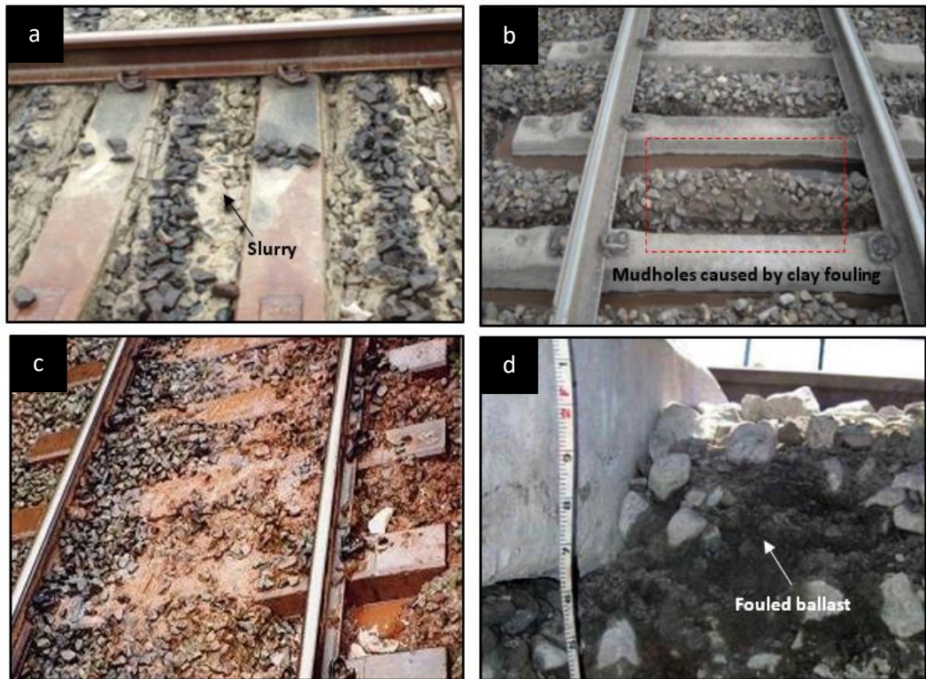
Figure 2. 1: Mud pumping sites in (a) Ashfield, New South Wales (Tennakoon et al. 2014) (b) Queensland (Indraratna et al. 2012), (c) The United Kingdom (Ghataora et al. 2017) and (d) Mansfield, Massachusetts (Aw 2007)
