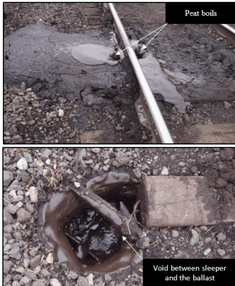
Figure 2. 8: Peat boils and voids between the sleeper and the ballast (after Wheeler et al. 2017)
