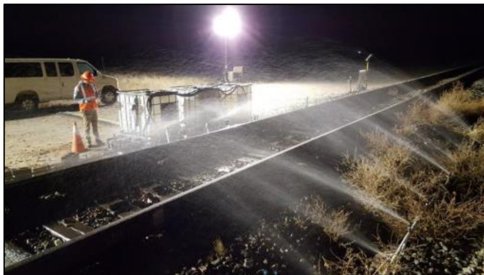
Figure 2. 7: Rainy test section with fouled ballast (Li & Wilk 2020)
