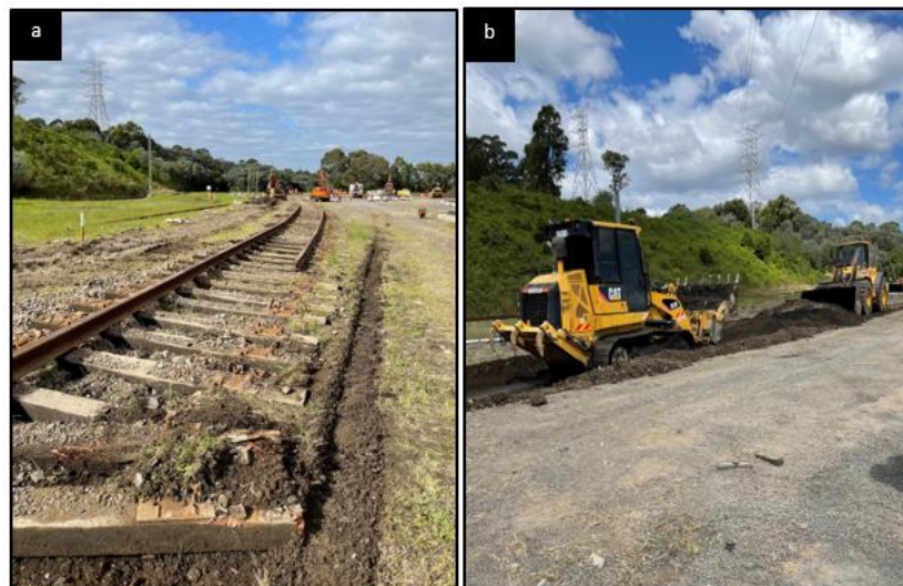
Figure 10. 3: (a) Existing track in Chullora, and (b) Excavation at the instrumented control section (ICS)
