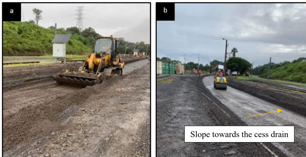
Figure 10. 20: Laying capping material on the drainage layer, and (b) Compaction of capping
