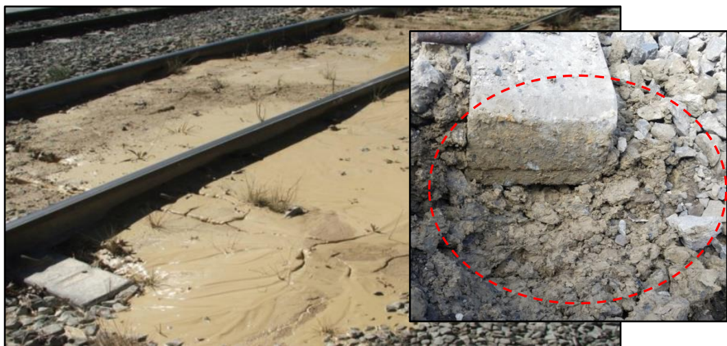
Figure 7. 1: Subgrade mud pumping and loss of contact between sleeper and ballast (Courtesy: Prof Buddhima Indraratna)
