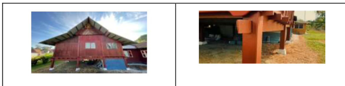
Fig. 14: A raised floor on stilts protects against flooding and animals. (Source: Author, 2022)
