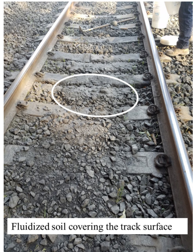
Fig. 1 Subgrade soil fluidized and migrated to the track surface (ballast contamination) as observed during site investigation in the Eastern coast of NSW
