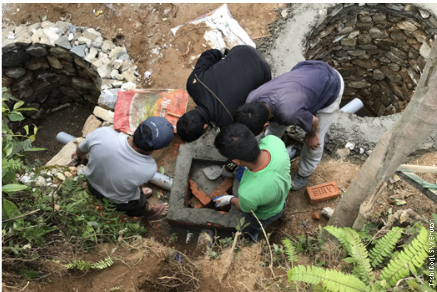
Figure 22. Installation of diversion chamber as an effective approach to safe faecal sludge management in rural communities.
