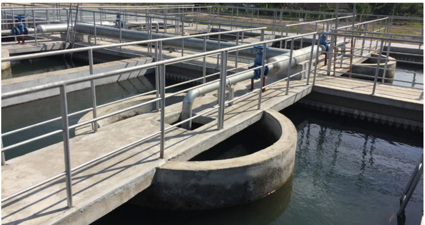
Long Thanh Water Scheme - part of climate-resilient water safety planning in Vietnam, where access to water is under extreme threat from a growing population, increasing demands of agriculture and industry, and the worsening impacts of climate change, including drought and floods Credit: Thrive Networks/East Meets West / Tran Tuan Anh
