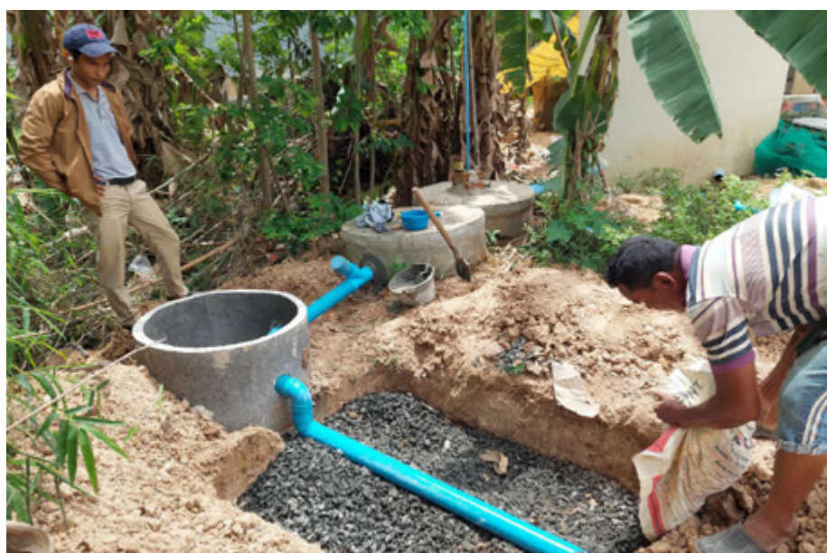
A sanitation business labourer installs an iDE-designed latrine upgrade to maintain toilet functionality in high groundwater and dense, saturated soil. He adds gravel to the leach field to provide preliminary treatment of the wastewater and increase surface area for improved infiltration
