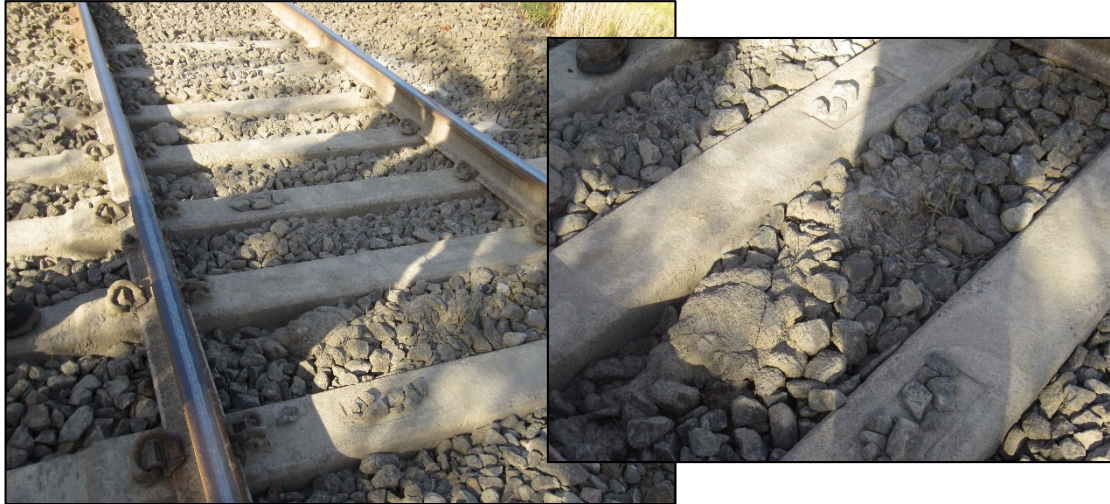
Figure 1: Subgrade mud pumping at Kembla Grange, NSW, Australia (Korkitsuntornsan 2020)
