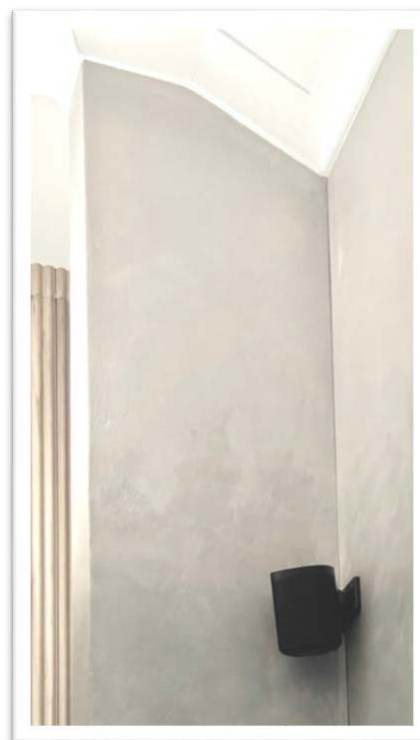
Figure 6.7 Sonos wall speakers above listener Sonos speaker on southern waiting room wall, three metres above seated patient, taking advantage of cathedral ceilings and a wide stereo field
