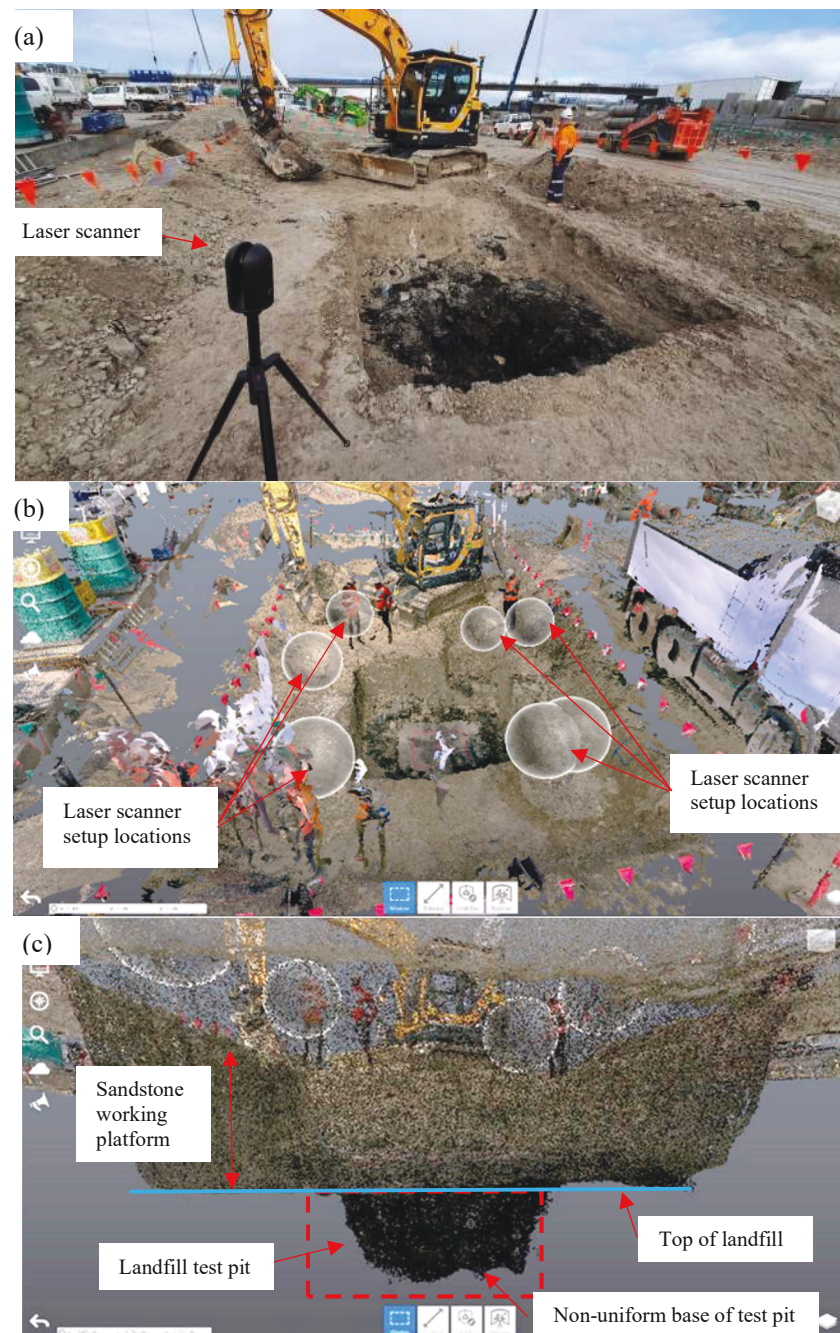
Figure 3.2 Test pitting at the landfill (a) Test pit excavation, (b) Overlaid point clouds from laser scanner viewed from Autodesk Recap software (note: white circles indicate location of laser scanner setup points to map the entire test pit, and (c) Elevation view of test pit capturing base of test pit excavation
