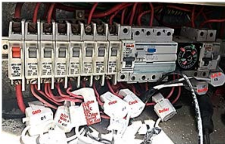
Figure 73: Eight Current Sensors from Smappee installed in the switching panel of a picogrid
