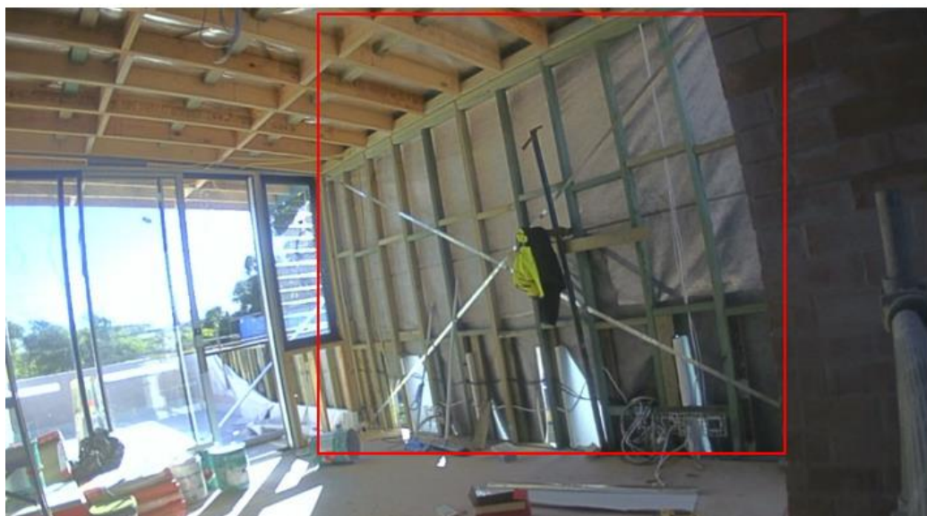
Figure 4.10: The slightly inclined region of interest captured by the camera
