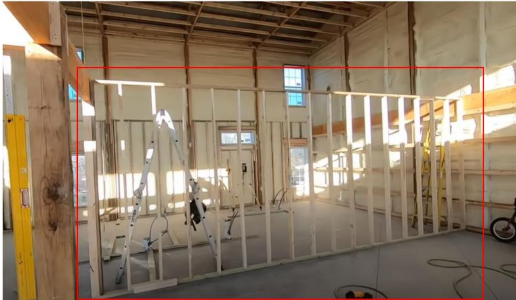
Figure 4.7: Backlight caused by natural light entering the site
