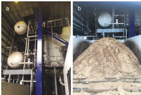
Fig. 3. (a) Existing biomass boiler and (b) biomass feedstock, photos taken by co-author Ximenes in 2021.
