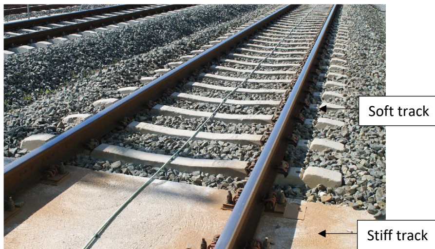
Figure 5.1: Track transition between ballasted track and slab track sections on the high-speed line Cordoba-Malaga, Spain, (Sañudo et al. 2016)
