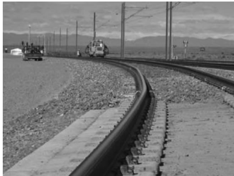
(b) Slab track to ballast track transitions indicating alignment error (Li et al. 2016)
