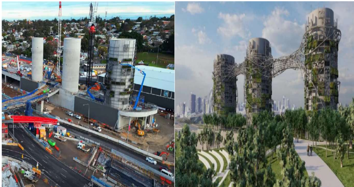
Figure 2. Tunnel ventilation stacks for the M4-M5 Link tunnel under construction and the final artist impression covered in green wall technology.
