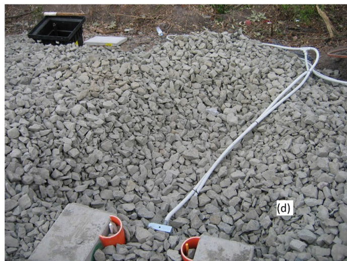
Fig. 16 Field instrumentation at Bulli: a Schematic of all instruments b Displacement transducer, c Settlement pegs d Protective casing for cables (modified after Indraratna et. al. [20])
