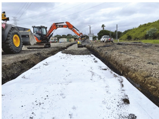
Figure 2. Geocomposite installation to mitigate the fluidization potential of soft soil at Chullora, New South Wales (an ongoing pilot study supported by Sydney Trains).
