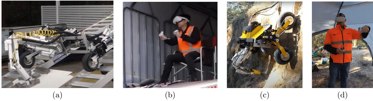
Figure 7: Field testing: a) In the car park by deploying HALO off a truck, (b) Operator is seated in the back of the truck, (c) Real-world trial at a sandstone quarry, (d) Operator is free to walk around within the command tent.
