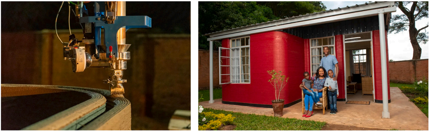
Fig. 10. 14Trees project: (a) printing process (b) completed building [152]. Image courtesy of the 14Trees.
