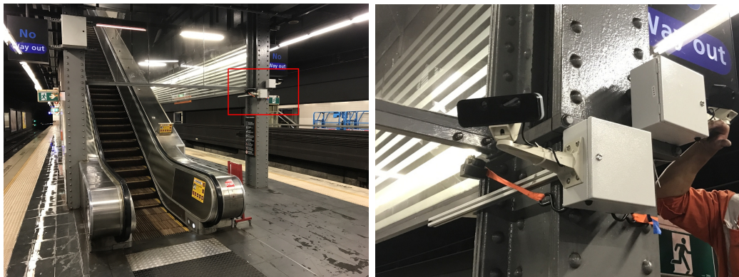
FIGURE 5.7: Early prototype systems installed on Town Hall platform 5/6 for data collection. Left image shows the location of system 2 and 3 from Figure 5.6. Right image shows a close up of system 2.
