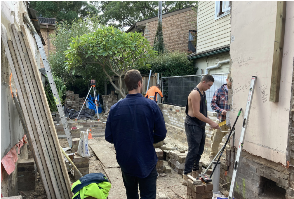
Photograph showing bricks recycled from demolition stockpiled at the rear of the site and being used in the construction of the building addition.
