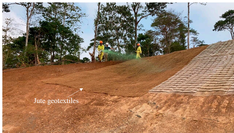
Figure 7. Using jute geotextiles for erosion control and slope stabilization (a practical project carried out in Vietnam, 2022–2023, photo provided by FUCON).
