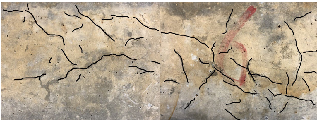
Figure 6.4 ASR cracking development and growth on the surface of prisms.
