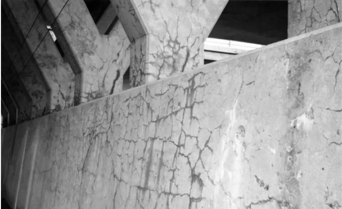
Figure 1.3 Multiple cracks on the surface of road over-pass pier. (Blight, 2011).
