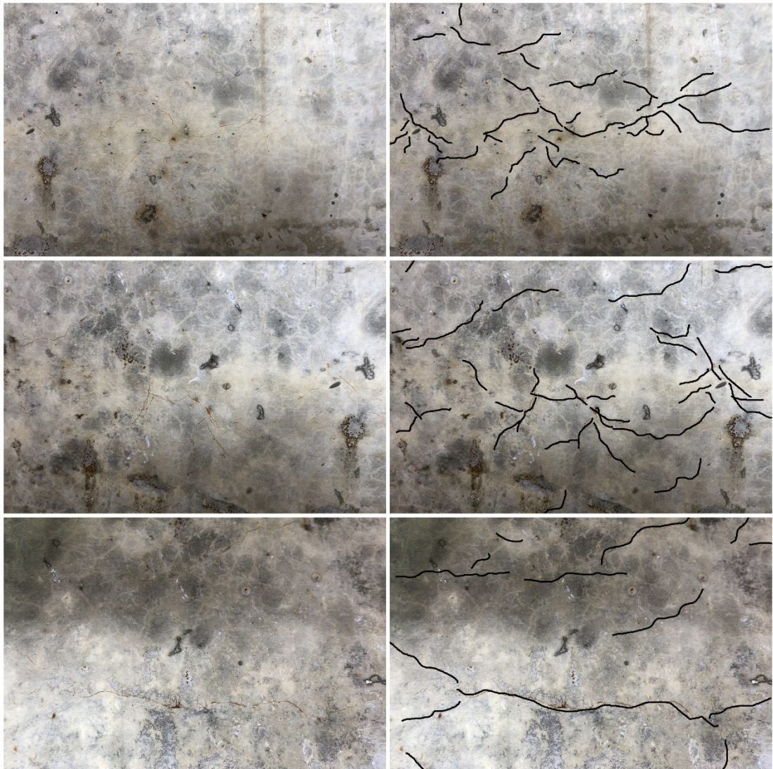
Figure 6.8 ASR cracks on the surface of reactive prestressed beams.
