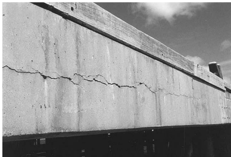
Figure 1.4 Longitudinal cracking of Prestressed jetty structure in Western Australia due to ASR (Cherry and Green 2021).
