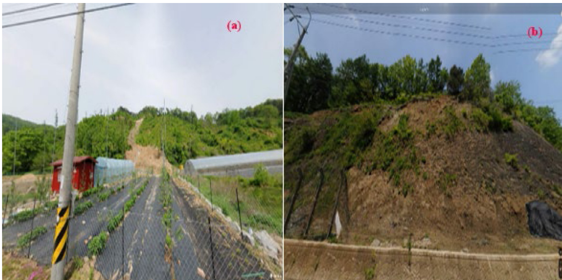
Fig. 3. Panoramic (a) and close-up view (b) of a landslide occurrence on July 16, 2018, in the Cheongju region ( 36^{\circ}40'18.58''\text{N} , 127^{\circ}42'3.28''\text{E} ).
