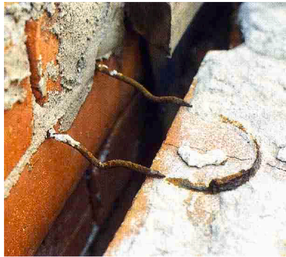
Fig. 2. Corrosion of the part of the tie embedded in mortar (Photograph taken by Prof. Adrian Page in 1989 the after Newcastle Earthquake).
