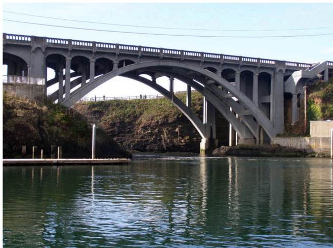
Fig. 13. Depoe Bay Bridge with thermally spayed zinc over the surface (picture from [56]).
