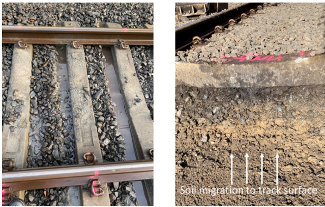
Water ponding and undrained condition due to track fouling at mud pumping spot
