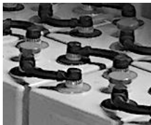
Figure 4.11 A Battery System
