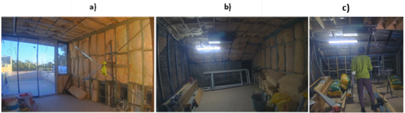
Fig. 2. Indoor location with a) Natural lighting; b) Artificial lighting c) Construction personnel and material creating occlusions.
