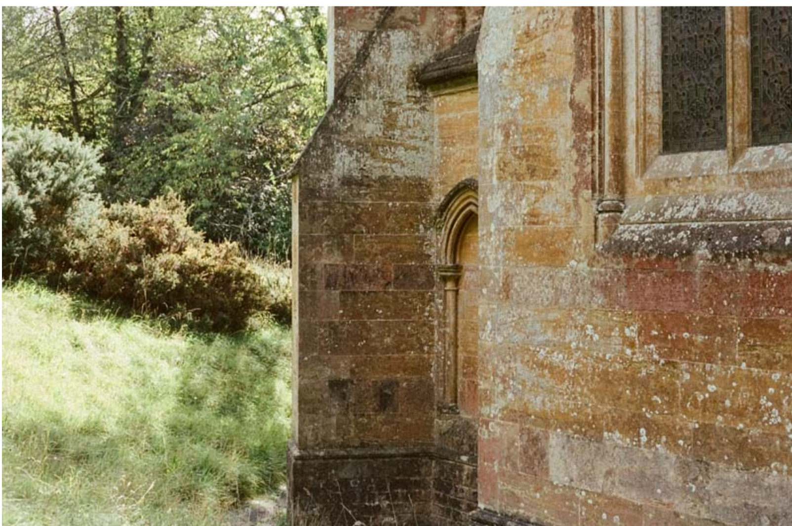
Fig. 13. Weathering on the Gibbs family chapel.
