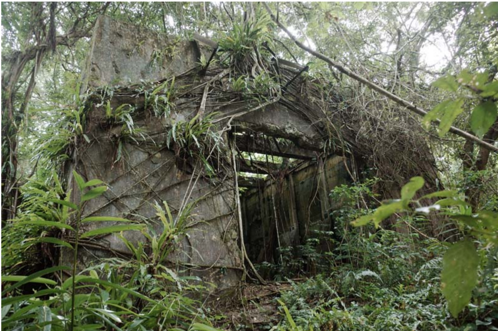
Fig. 18 – The entry to the concrete phosphate storage bin, located directly next to the ruins of the Gute Hoffnungshütte.
