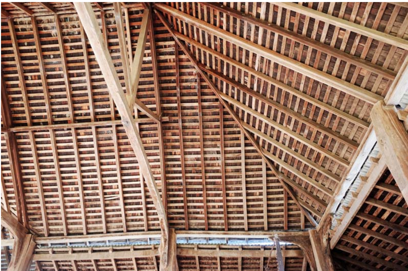
Fig. 11. The fine detailing of the Blacket Barn plays a central role in Tocal's state heritage listing.
