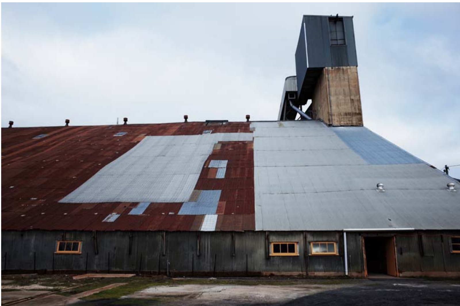
Fig. 30. The exterior of the Murtoa Stick Shed. Light passes into the interior through thousands of old screw holes in the metal roof sheeting.
