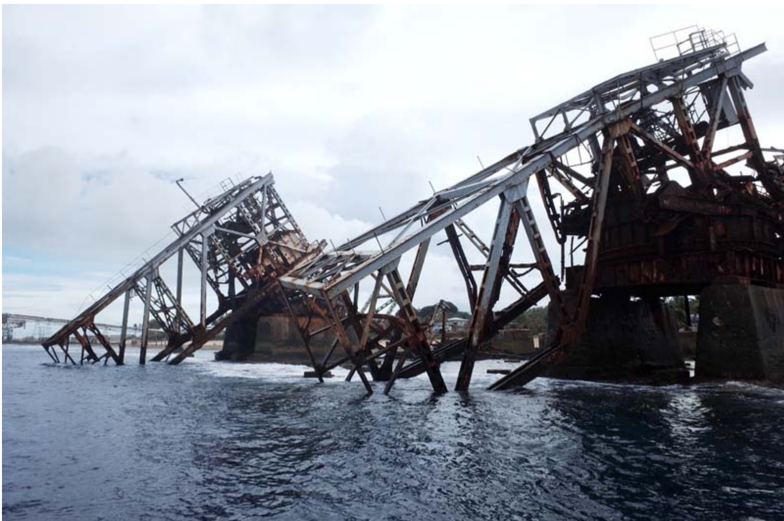
Fig. 20. The BPC's steel cantilevers sit collapsed onto the coral reef, surprisingly intact given the corrosive environment and heavy seas they face.
