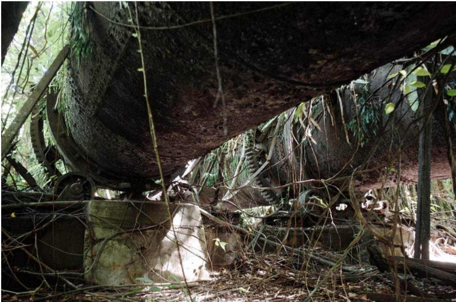
Fig. 14 - The undersides of the rotary driers used to reduce the moisture content of the phosphate prior to export. White phosphate was still stuck to the insides of the drums, seventy years after mining ceased.
