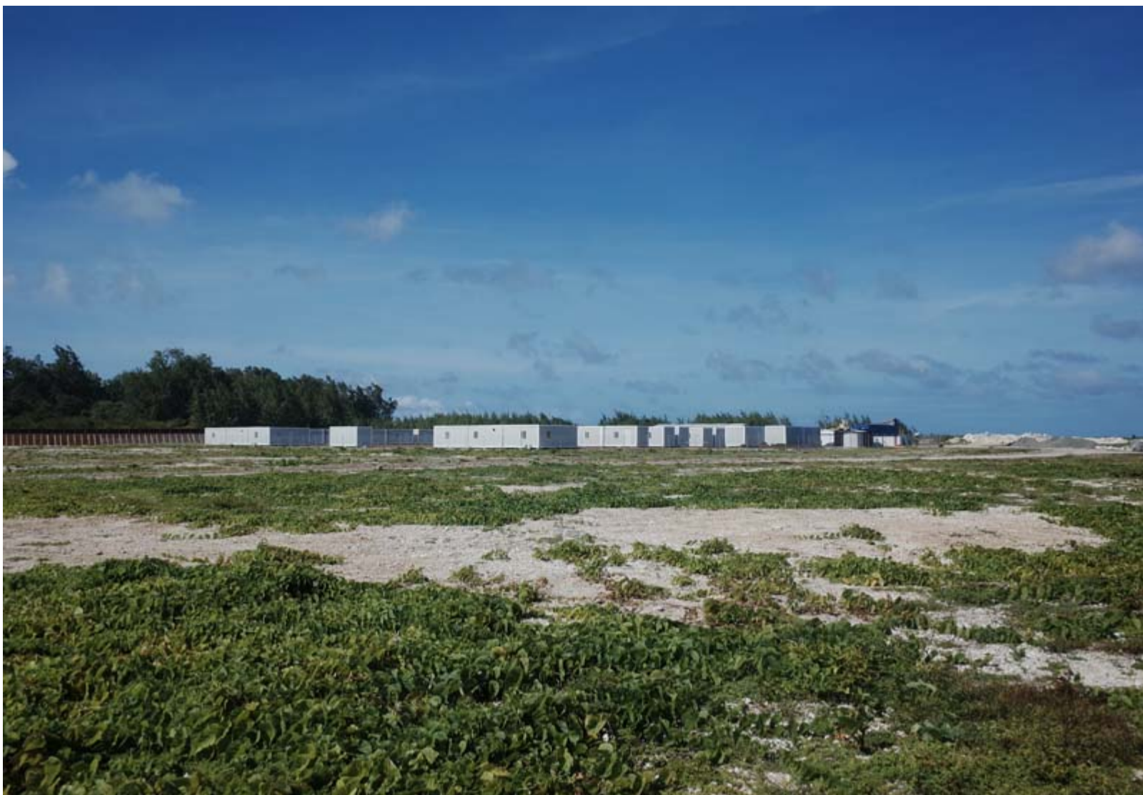
Fig. 26 – The surveillance station currently being constructed adjacent to the landing strip on Angaur as part of the US Air Domain Awareness Program.
