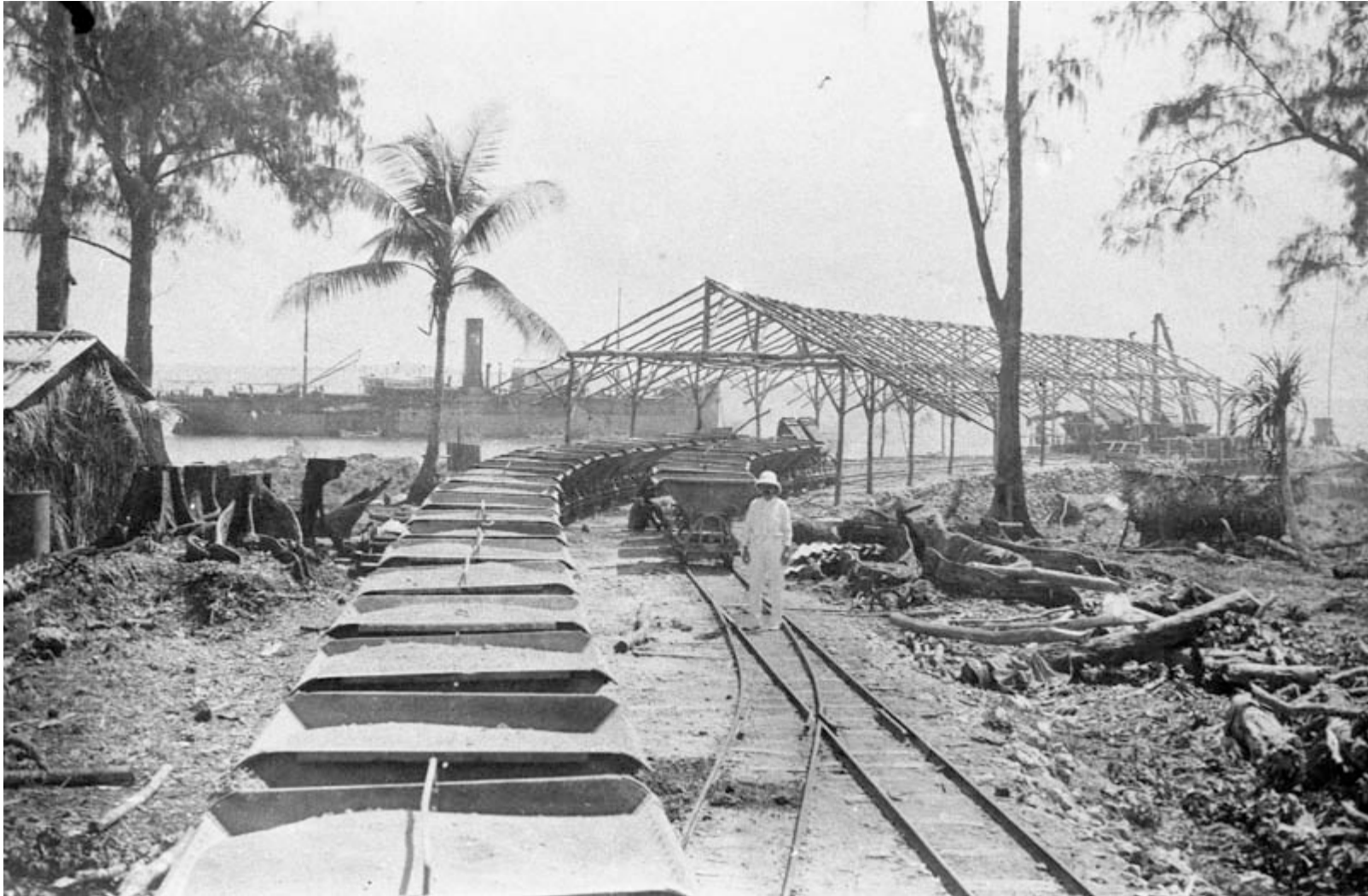
Fig. 32. Preliminary tracks, carts and loading equipment on Angaur, provided to the Deutsche Südseephosphat Aktiengesellschaft by F. H. Schmidt. A Lloyd steamer waits to be loaded in the background, c.1908. Source: Deutsches Bundesarchiv, Sammlung Heinrich Hagedorn, Bild 223-046.
