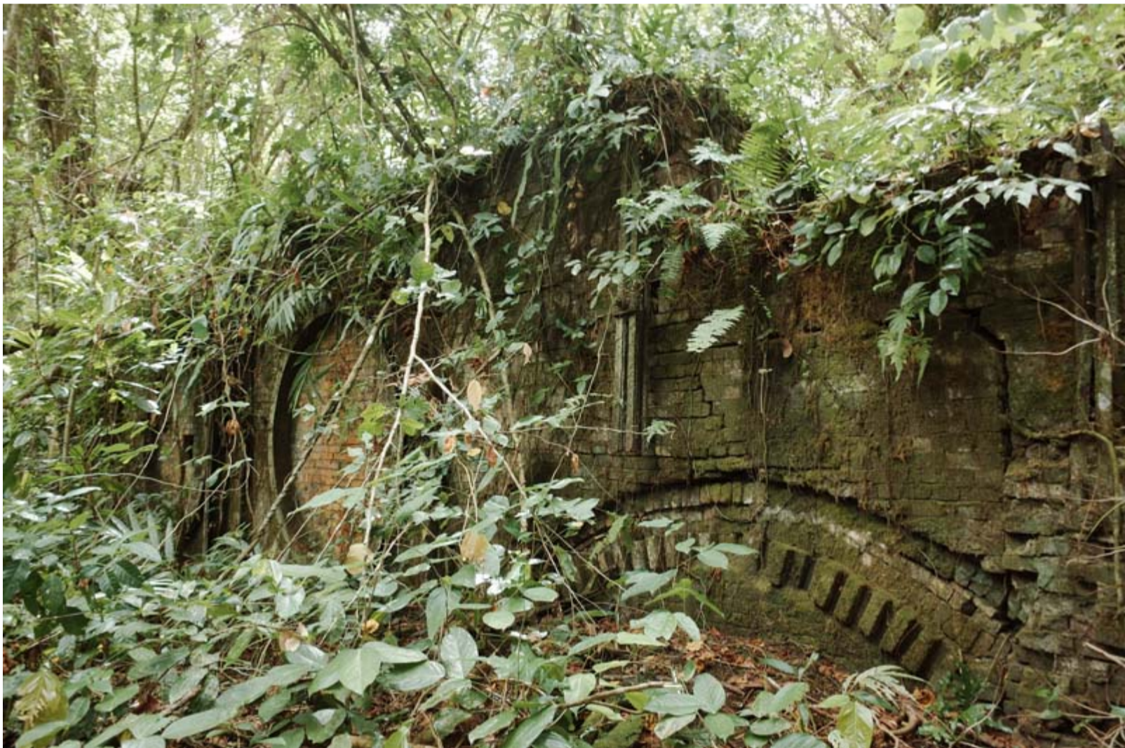
Fig. 16 – A brick kiln, built by the DSPAG and used to heat the rotary driers shown in figure 14, threatens collapse. The circular shape to the left of the image is the manifold that was used to attach the drums to the kiln.
