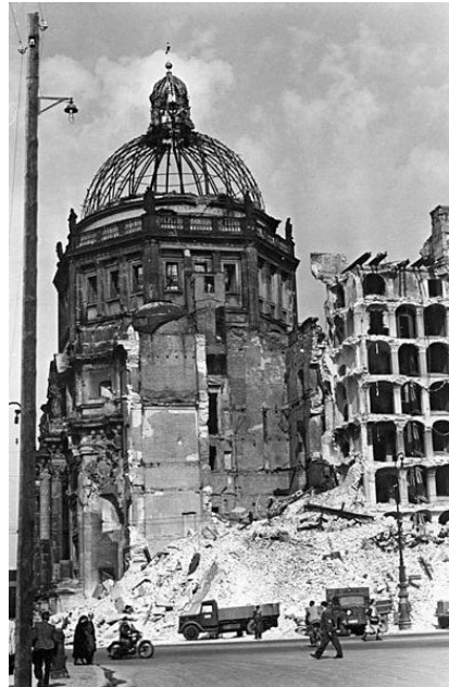
Figure 1. The Stadtschloss during demolition, 1950. Photographer: unknown. Image courtesy of the Deutsches Bundesarchiv (Bundesarchiv Bild 183-07964-0001; Creative Commons CC-BY-SA 3.0).
