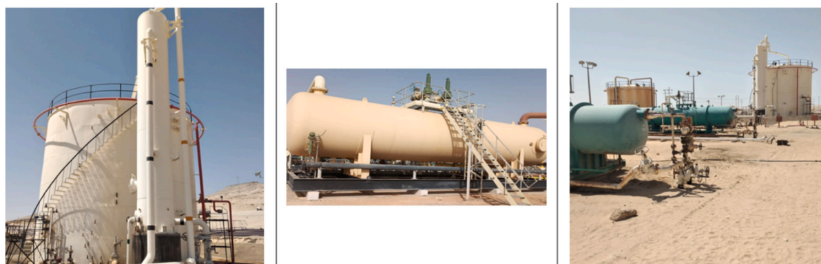
Fig. 1. Production operation system- Oil field – Libya 2024.
