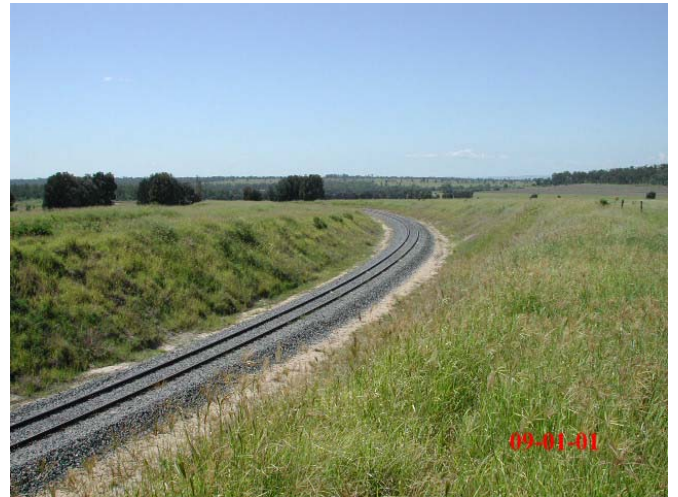
Figure 8. Boundary Hill Site. Drip lines were laid on all batter sections at row spacing between 1 m and 2 m.
