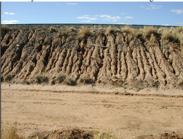
Laleham Site: rill erosion on an embankment batter
