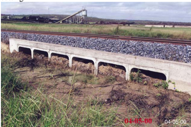
Boundary Hill Site: eroded sediments chocking culverts
