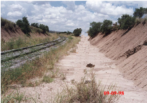
Boundary Hill Site: eroded sediments fouling ballast in a cutting
