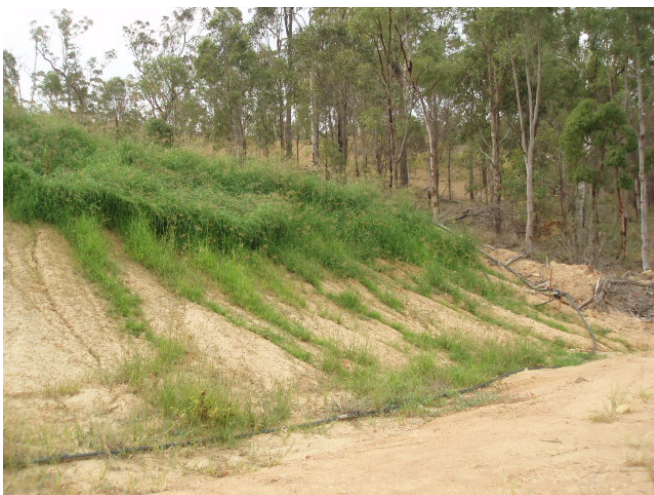
Figure 13. Holmes cutting – four rows (1 m spacing) of drip lines were laid at the top section only.
