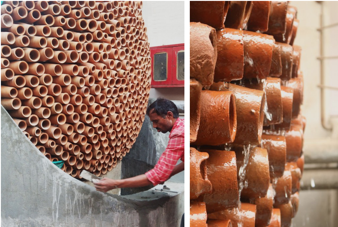
Figure 6.3. Deki Cooling Installation, Ant Studio (2017). A terracotta cooling installation installed in Uttar Pradesh, India.
