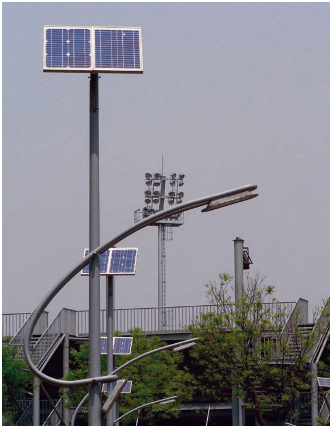
Streetlamp with photovoltaic panels on its top at the Fengtai Softball Field.
