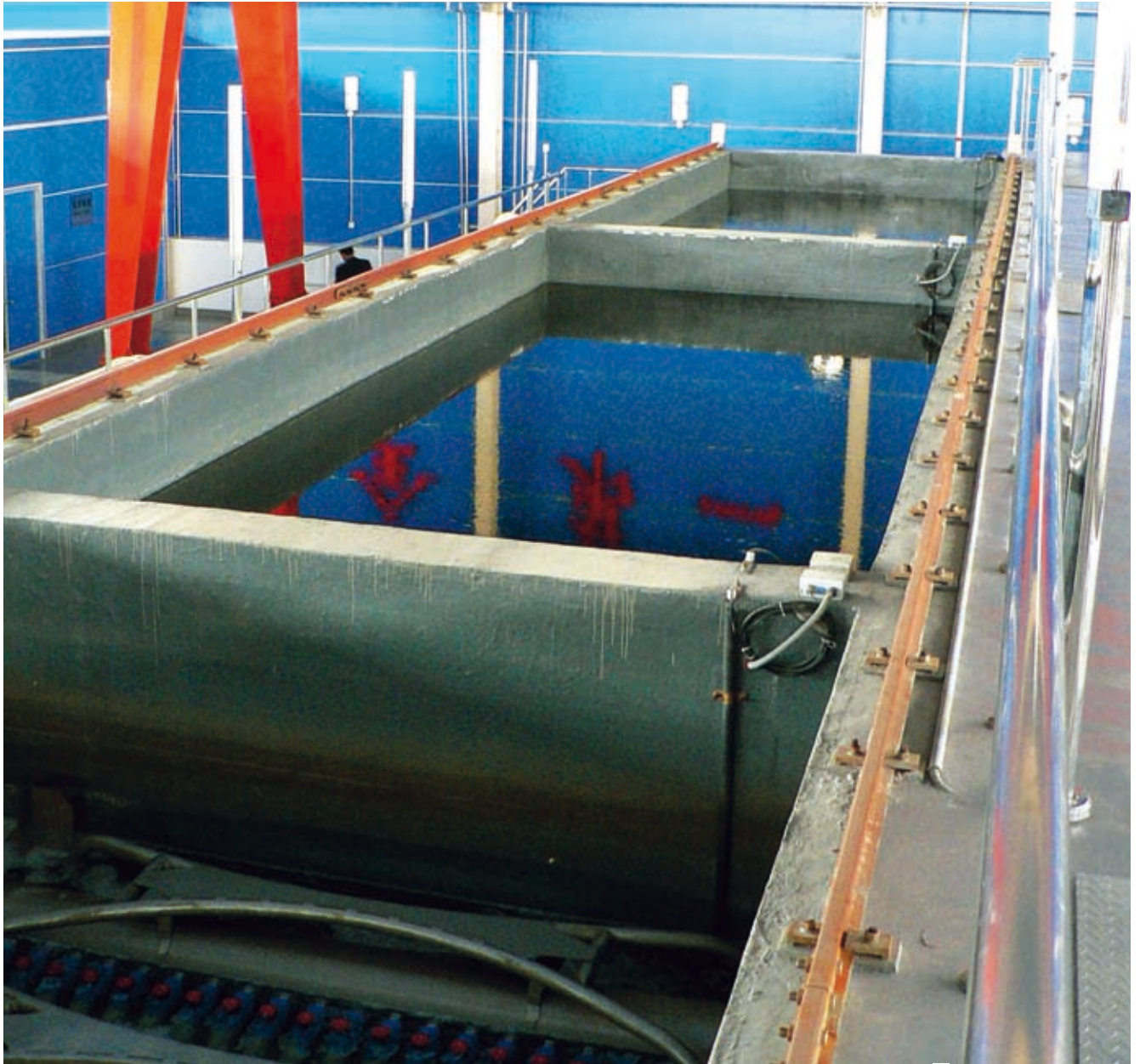
Wastewater Treatment process at the Qinghe Reclaimed Water Plant
