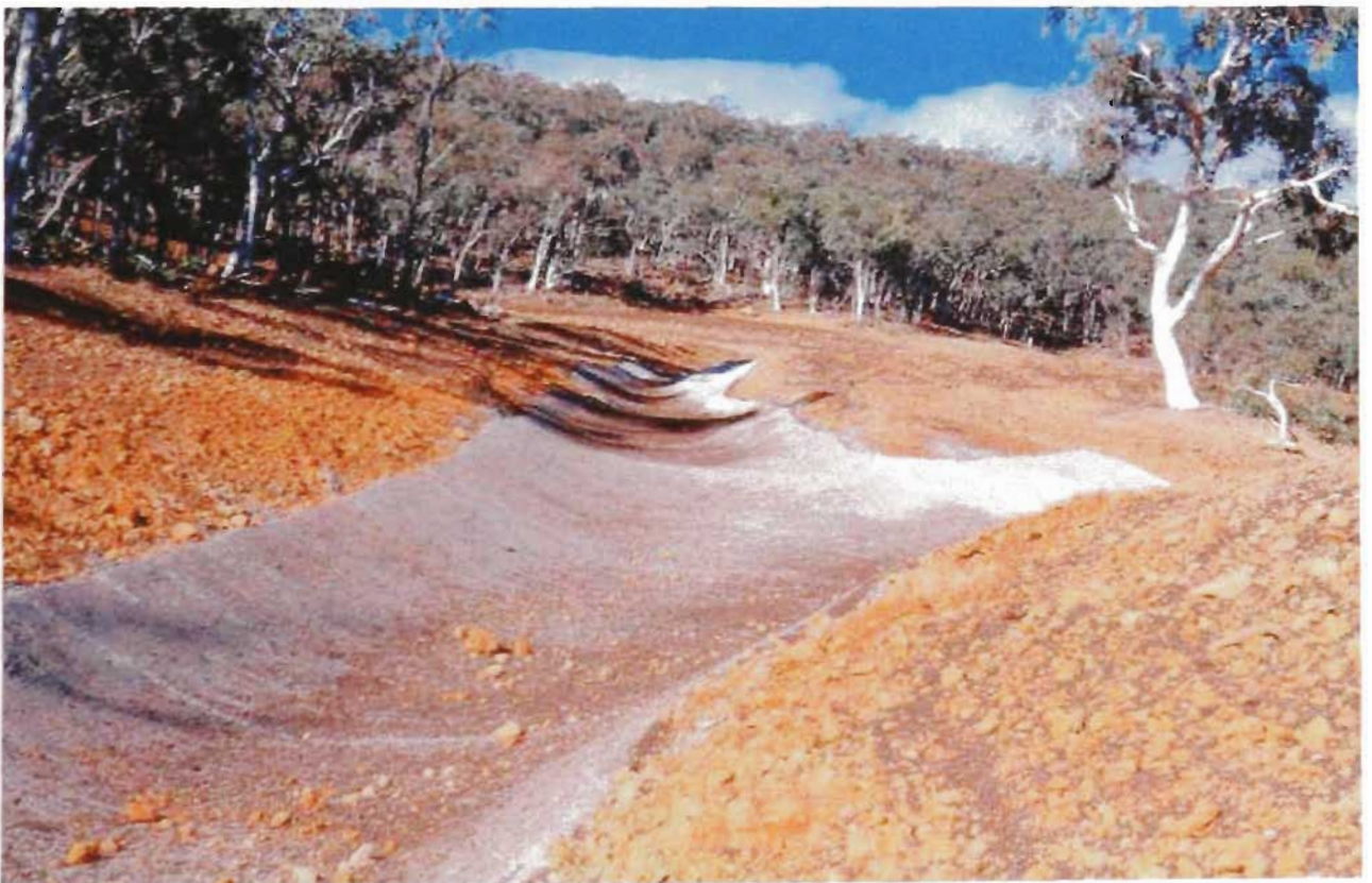
Figure 4.7 Remediation at Mt. Costigan: concrete culvert. Viewed towards the west. Patchy biosolid is visible to the right of the culvert.
