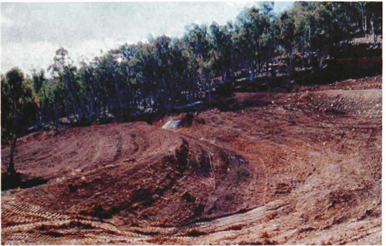
Figure 4.6 Remediation at Mt. Costigan: soil terraces and berms. Barren site, viewed towards the north.
