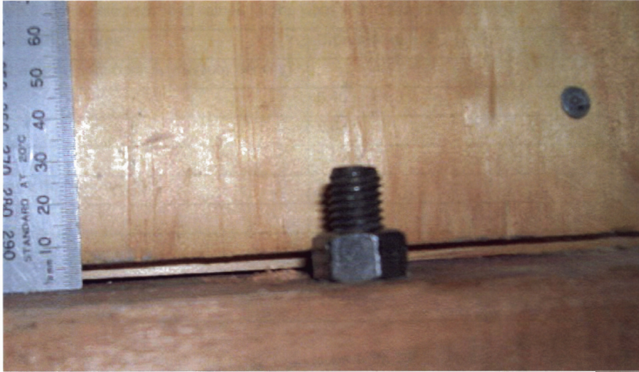
Figure 5.7 A gap of 5 mm on the far end wall.
