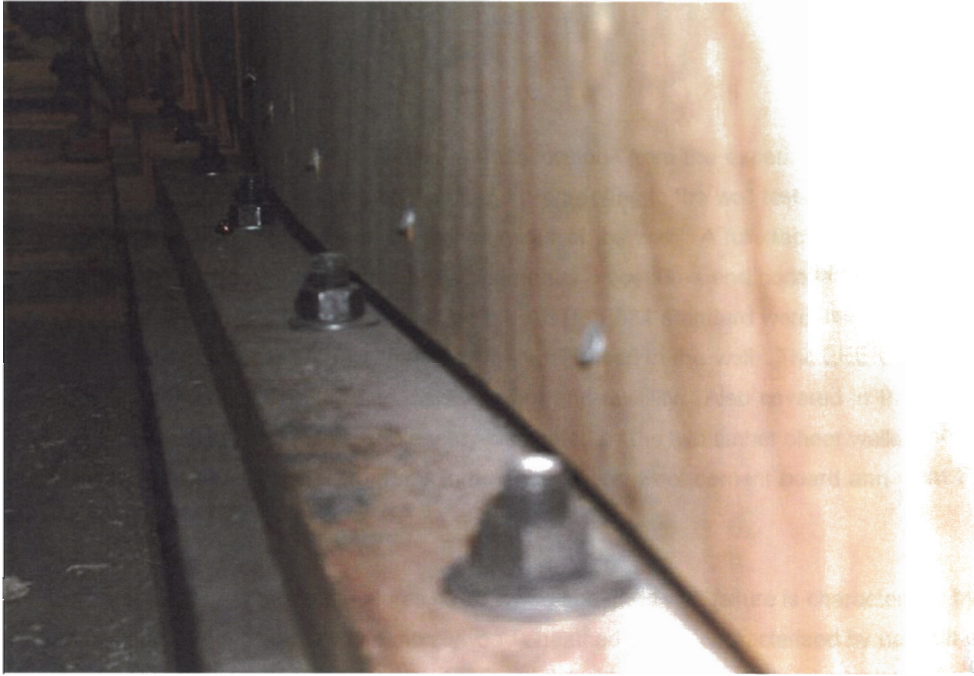
Figure 5.13 Nail pull-out starts from the base where top load is applied.
