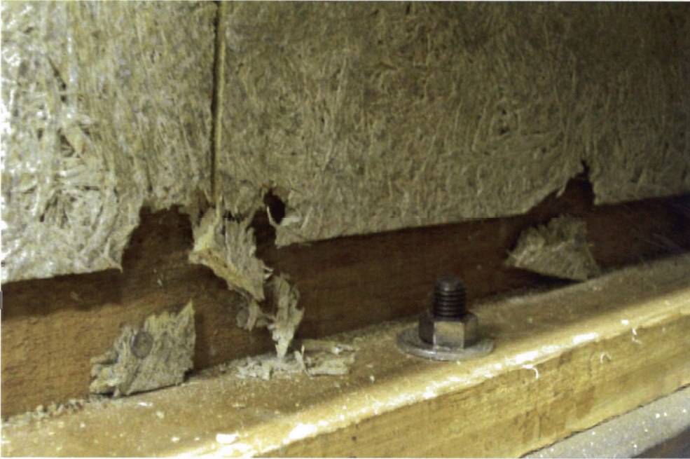
Figure 5.8 Tearing of the nails through the walc panels.
