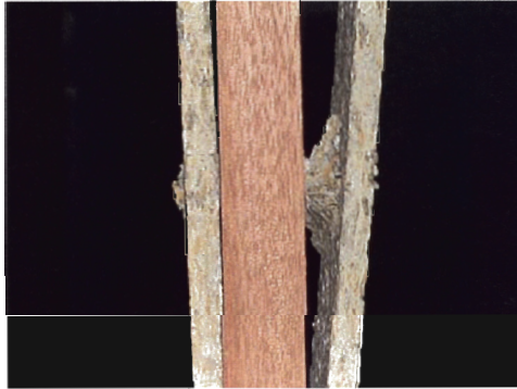
Figure 5.1 Nail tear through the wwcb.
