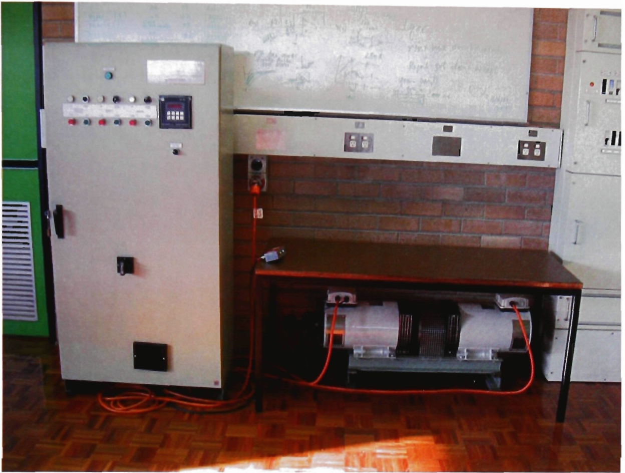
Figure 5.1: The Static VAR Compensator (SVC) system.
