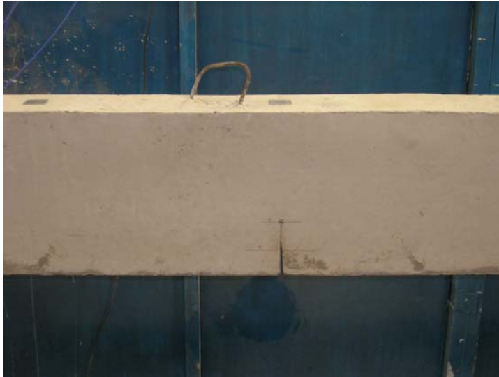
Figure 7.4 An elevation of a typical inflicted crack damage
