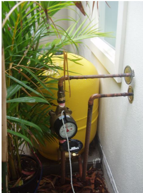
Figure 5-7 Example of a large domestic pressure vessel used as part of a rainwater supply system
