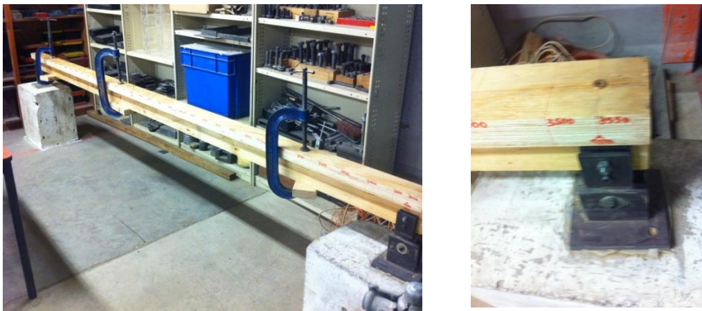
(d) Clamping of flange and web before screwing (e) Installation of screw
