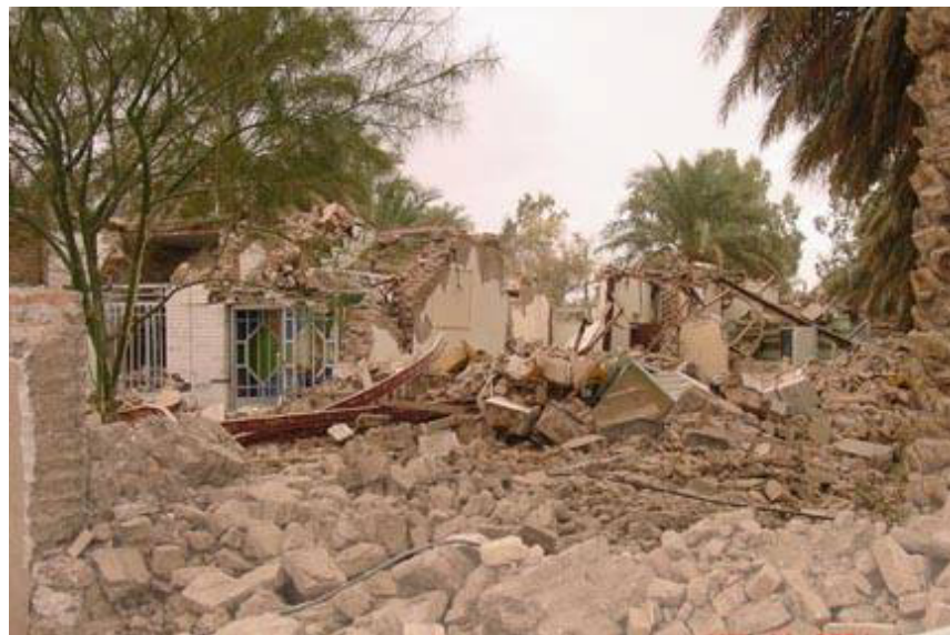
Figure 1.8: Collapsed Adobe structures by Bam Earthquake Jan 14, 2004 (World Housing Encyclopedia).
