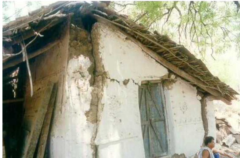
Figure 3.7: Cracking and separation of walls in 1997 Jabalpur Earthquake (Source: World housing Encyclopedia, reports # 23).
