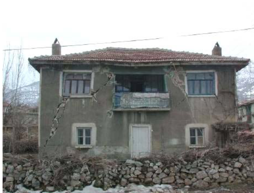
Figure 3.5: Inclined cracking in the wall in Pinarkaya. (Source: GFZ-German Research Centre for Geosciences)
