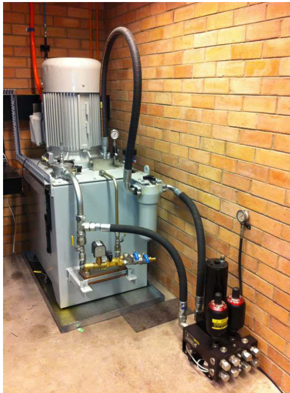
Figure 6.4. One motor-pump unit of the test rig
